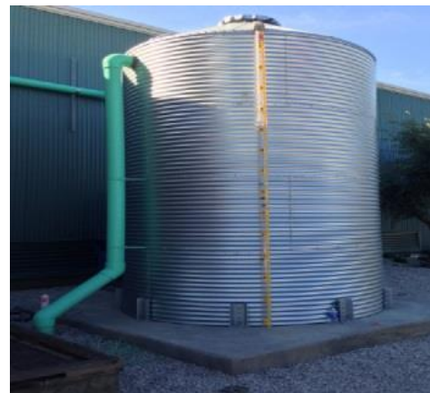
RAINWATER HARVESTING CISTERN, ENVIRONMENTAL INNOVATION CENTER, SAN JOSÉ
