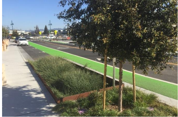
BIORETENTION AREA IN CONCRETE BOX WITH UNDERDRAIN, EMERYVILLE, CA (SOURCE: EOA, INC.)
