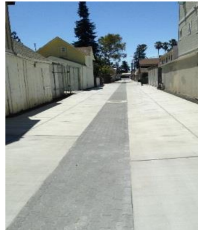
INFILTRATION TRENCH WITH PERVIOUS PAVEMENT, SAN JOSE (SOURCE: CITY OF SAN JOSE)
